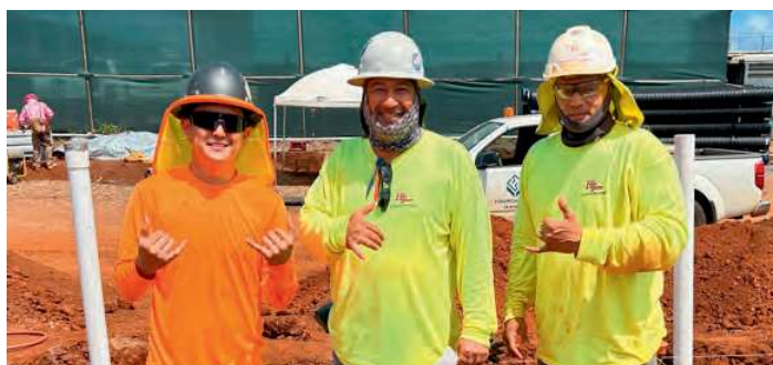
Rice Street Apartments. Hi Tech Plumbing. GC: Unlimited Construction (l-r) Victor Yi, Duke Mier, Charles Hokoana.
