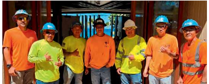
Mauna Kea Beach Wing Renovation. Dorvin D. Leis. GC: Nordic PCL. (l-r) Aaron Correa, Jay Omori, CJ Ancheta, Dave Paoa, Kyle Tsukamoto, Aden Cabalce-Agno, Abe Vallente.
