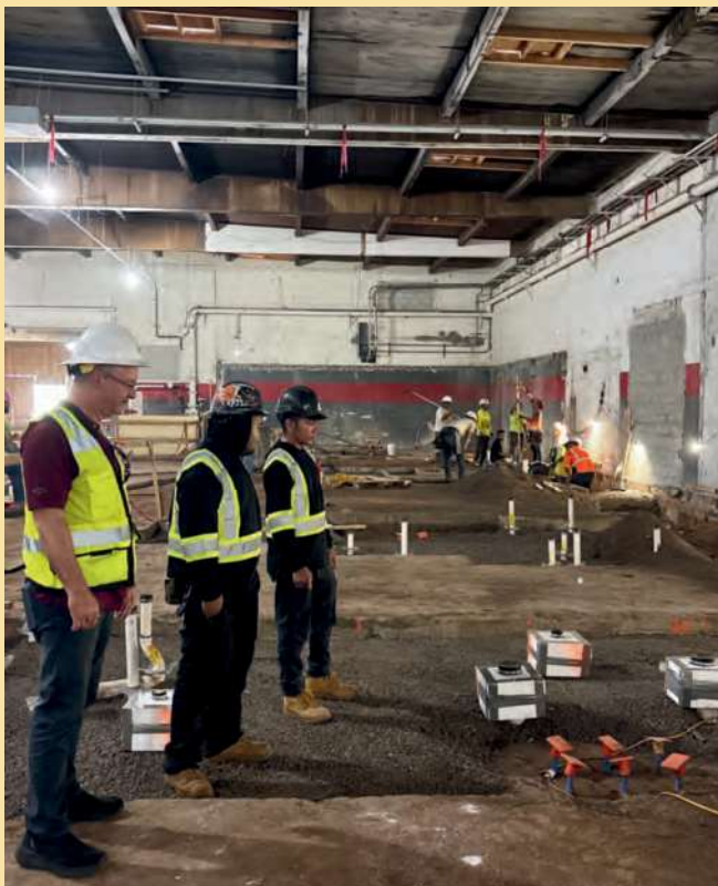
President Matthew Brady, with Journeyman Anthony Edrado and Apprentice Zachary Clemente from Alakai Mechanical, conducting a pre-pour check for the cement at the New Union Building in Aiea.
