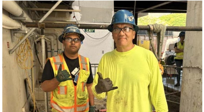
Queens Emergency Room Renovation. Dorvin D. Leis. (l-r) Jansen Fujinaga, Keawekulooa Leong. (GC: Hawaiian Dredging)
