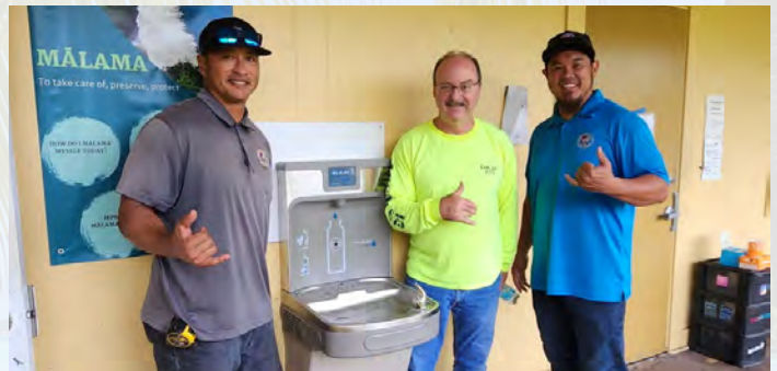
Business Agents installed a water cooler with a water bottle filler between classrooms in one of the school buildings at Pahoa High School. (l-r) Sam Barrett, Jr., Matt Brady, Sheung Man Wong.
