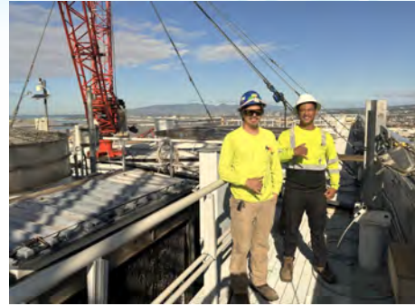
First Hawaiian Bank Cooling Tower Replacement. Oahu Plumbing. GC: Nordic PCL. (l-r) Kristopher Gellert, Ezekiel Telea.
