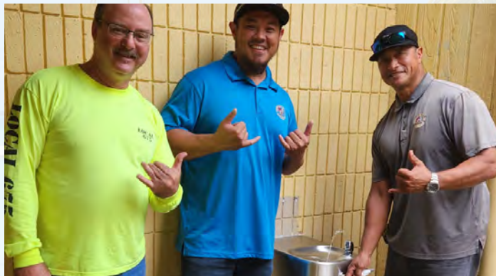
Business Agents Matt Brady, Sheung Man Wong, and Sam Barrett, Jr. volunteered their time and installed a water fountain outside Pahoa High School's cafeteria as part of "The Labor of Love" project.
