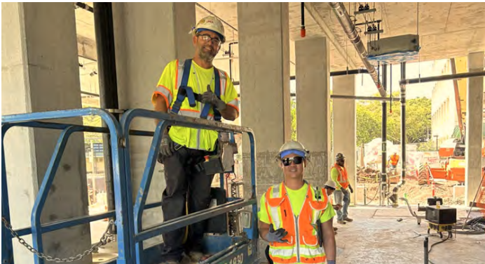
UH Manoa's The Residences. Commercial Plumbing. GC: Swinerton. (l-r) Roy Dunlap, Jared Matsumoto.
