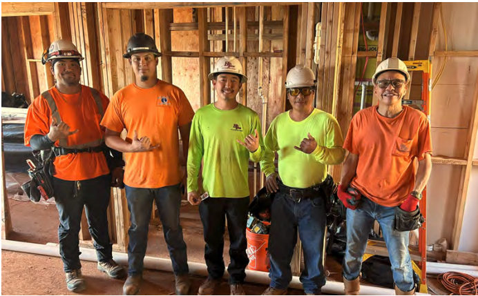
Kai Olino. Honolulu Fire. Hi-Tech Plumbing Corp. GC: Unlimited Construction. (l-r) Honolulu Fire: Danny Sugita, Allen Ucker. Hi-Tech Plumbing: Victor Yi, Cris Alvaro, Clif Murakawa.
