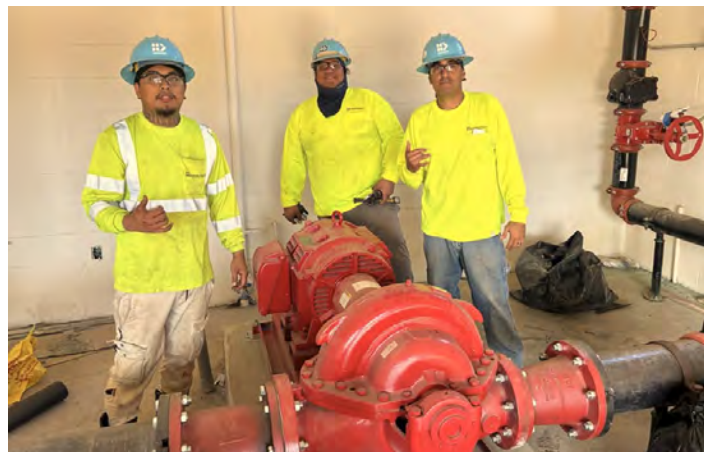
Honouliuli WWTP. Hawaiian Dredging Fire Sprinkler. GC: Hawaiian Dredging. (l-r) Isaiah Taumua, Keola Silva, Jensen Mata.
