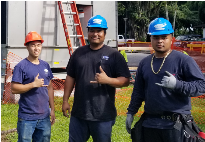
(l-r) Justin Kesterman (Apprentice), Leo Duropan (Working Foreman), Alain Rivera (Maintenance worker). Carrier Corp. Hilo Hawaiian Hotel Cooling Tower Changeout and HVAC Piping Project.
