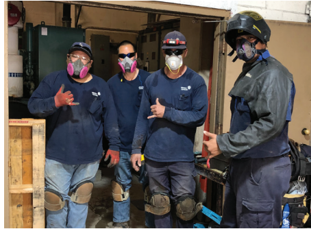
(l-r) Kawika Johnson, Scott Chun, Shane Kano, Ian Aoyama. Chiller Changeout, Discovery Bay Condominium. Johnson Controls.
