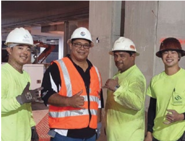
Nakamura Plumbing's Sean Tamayoshi, Sean Tania and Kyle Lau on Ewa expansion at Ala Moana Center.
