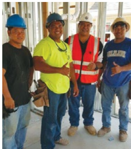
Nakamura Plumbing's Lance Takara, Dwayne Pagente and Shane Pagente on Hoakalei jobsite in Ewa.
