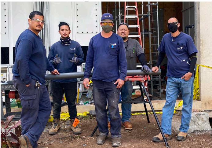
(l-r) Kawika Johnson, Kanai Aglipay, Scott Chun, Ian Aoyama, Shane Kano. Johnson Controls. Honolulu Park Place Cooling Tower Replacements.
