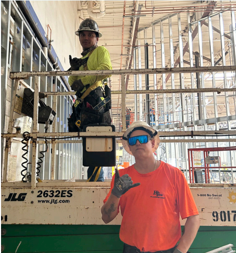
Ryan Torino (on the left), and Michael Malabon. Hi-Tech Plumbing. Seafood City Jobsite, Kahului, Maui.
