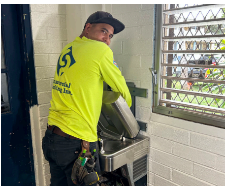
Jared Solidum with Commercial Plumbing installing the water fountain in the cafeteria.
