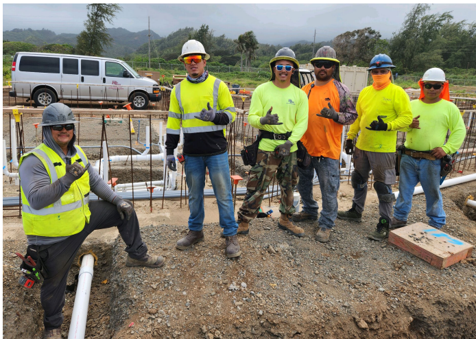
(l-r) Stephen Brissette, Bronson Abrazado, Keaton Carvalho, Reid Ogata, Charles Hokoana, and Cris Alvaro. Hi-Tech Plumbing. Brigham Young University Hales #11-13. GC: Okland Construction.
