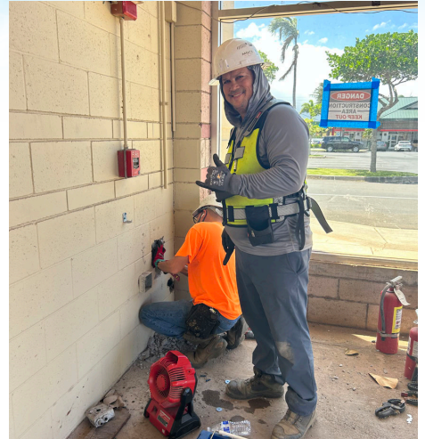
Stephen Brissette (standing), and Clifton Murakawa. Hi-Tech Plumbing. Seafood City Jobsite, Kahului, Maui.
