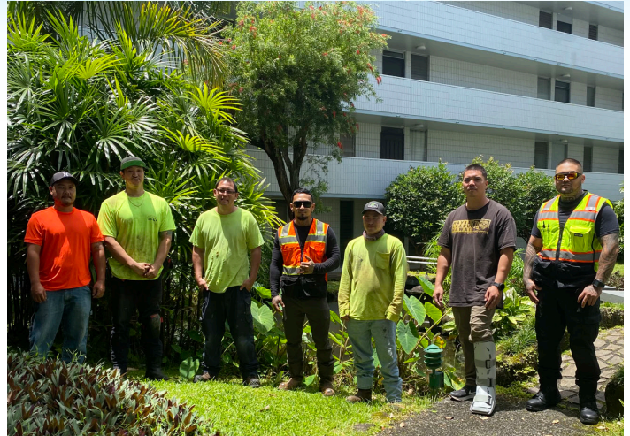
(l-r) Elson Lapot, Justin Imura, James Matsumura, Payne Williams, Shaun Takayama, Justin Dano, and Gareth Matutino Jr. Construction Management Services. Kunawai Terrace, DWV replacement.
