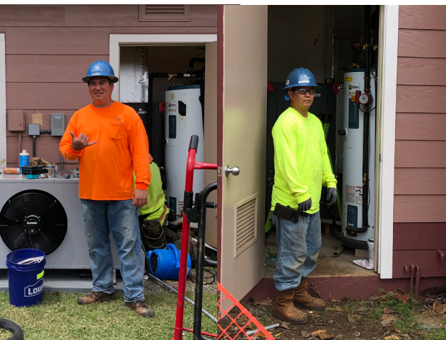
(l-r) Rex Tyau and Ryan Higaki. Geothermal Heat Pumps. Aliamanu Military Reservation. Dorvin Leis Co. GC: Actus
