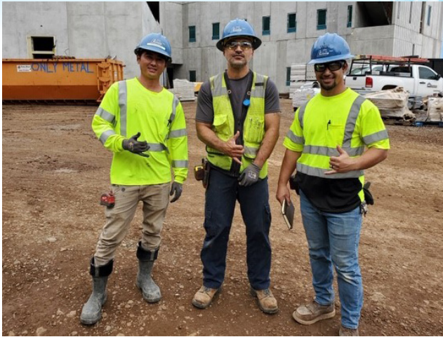
(l-r) Sean Sugihara, David Rapozo, and Keanu Solidum. Hawaii State Hospital, New Patient Facility. Dorvin Leis Co. GC: Hensel Phelps.
