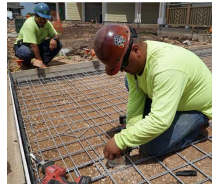
Jonah Hamada with TNH Plumbing working on leveling clean-out in the driveway of a single-family home.
