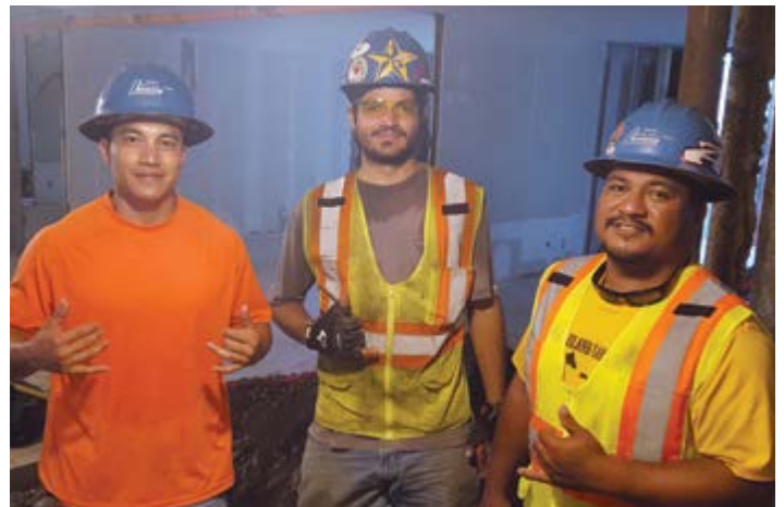
Dorvin Leis plumbers Jarren Tsukamoto, Cody Haddin and Sherman Martines on the Marriott project in Waikoloa.
