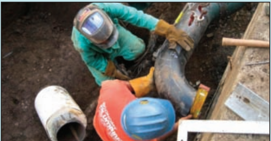
Local 675 workers on the job at the ongoing Maryknoll School gymnasium project due for completion later this year. At top, Continental Mechanical apprentice Shane Oshiro is threading pipe, and below, journeymen Michael Yamada and Randall Matsuzaki, of Economy Plumbing, prepare the underground piping to tie into the chill water piping on the other side of the wall.
